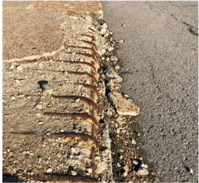
Figure 2: Concrete Cracking and Delamination Caused by Corrosion of Steel Reinforcement
