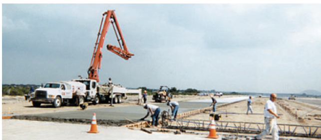
Point Mugu Naval Air Station required a 565-foot long, non-jointed pour of 30% Class F fly ash concrete.
